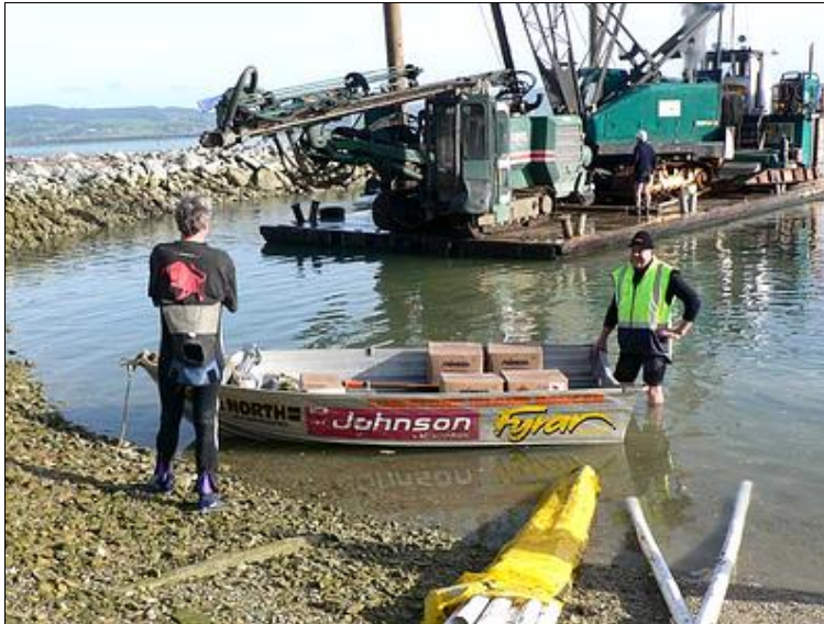
Wayne casually waiting for the drilling rig to manoeuvre into place with 6 boxes of plastic explosive in the dinghy!
