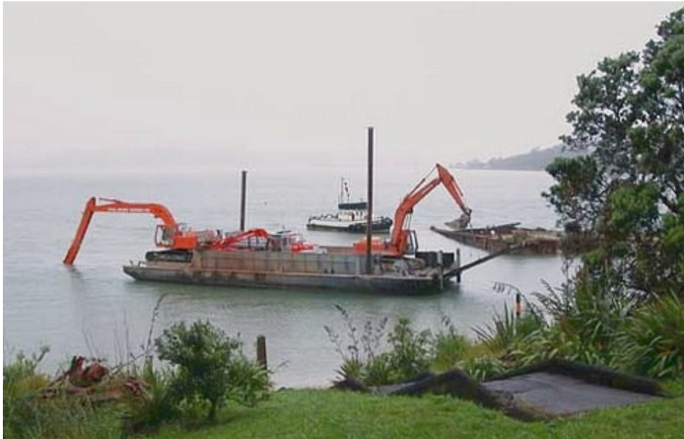
Heavy equipment arriving for the all tide berth construction – the new tractor squeezed in one corner!
